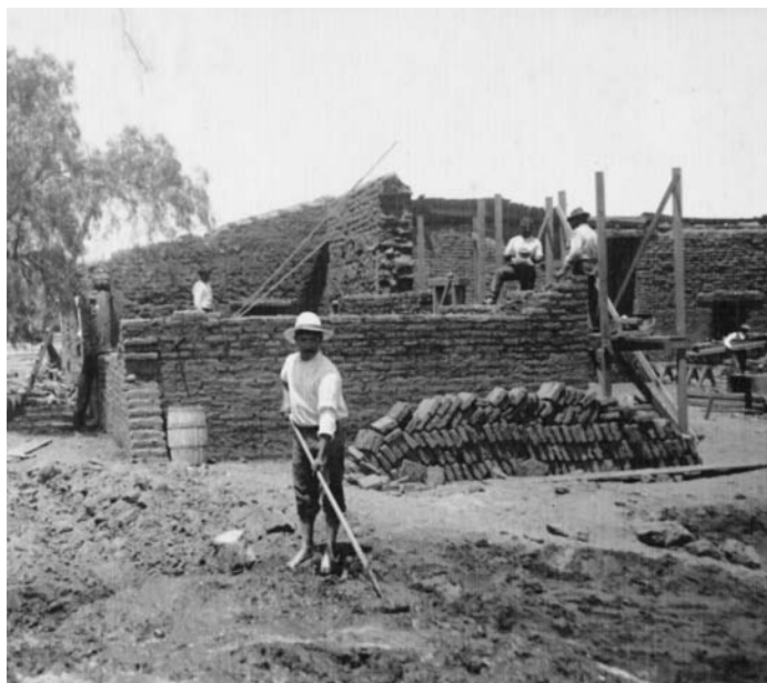
Figure 9: This photograph of the reconstruction of the Estudillo House shows Mexican and Indian workers making adobe bricks and assembling the walls. The two men in the background are identified as Romero and Mendoza.
